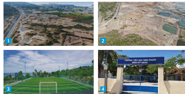
1, 2 - Van Phong Project 1 - Gravel on Landfill 3, 4 - Van Phong Project 1 - Futsal Court Construction and School Facility Repair
